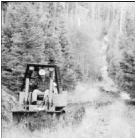
Chuck Horner operating the SWECO machine on new trail construction on the North Rim
